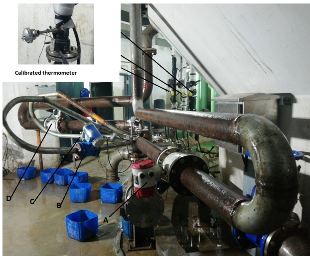
Figure 3: Flow meter and thermometer arrangement at cooling water pipes
