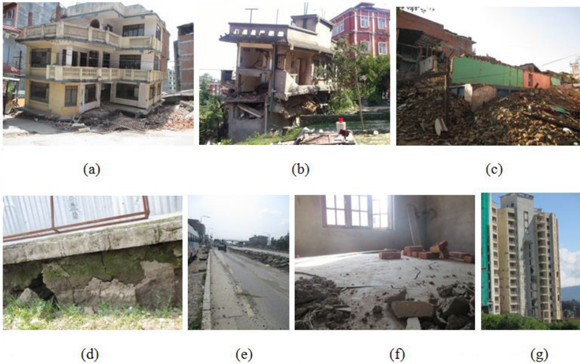
Figure 1: Some of the major destructions in Kathmandu valley. Figure (1a-1c) complete collapsed buildings in Gongabu, Balkhu and Sankhu area respectively. Figure 1d and 1e is the subsidence and displacement of the ground in Kausaltar area of Bhaktapur, Figure 1f shows the buckled floor in the newly constructed building in Balaju area and destruction in the apartments of horizon in Dhapasi area (Figure 1g)
