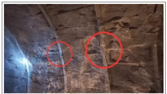
Figure 1: Buckling of Steel Rib on crown right wall of upstream of headrace tunnel.
