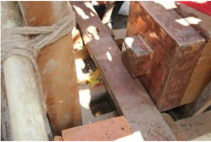
Figure 8: Ground floor thams provided with copper shoe (Source: Author)
