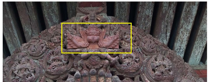
Figure 10: Head of Garuda repaired with new one on Southern (front) Tunda (Source: Author)
