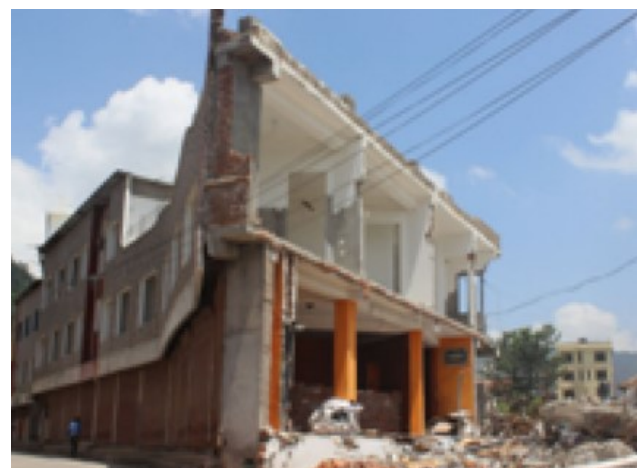
Figure 1: Non-orthogonal frame commercial building with severe damage in Kathmandu [3]
