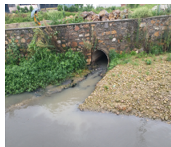
Figure 7: Direct drainage water at Segment-2 Source: Author
