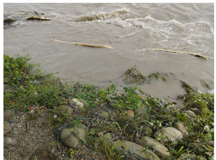
Figure 9: East Rapti River Eroding the Dike near Girijachowk
