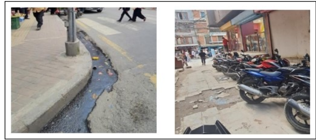
Figure 5: Hurdles due to broken pavement
