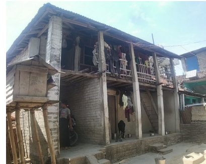
Figure 7: Addition of pillar and concrete block in old mud structure; Residence of Mr. Raj Kumar Chaudhary
