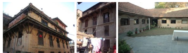
Figure 5: Photographs of Traditional homes, The inn and Yala Maya Kendra before adaptation
