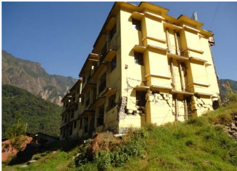
Figure 1: Damages on Buildings During to Sikkim Earthquake
