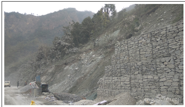
Figure 2: Hill side cut slope of Narayanghat-Mugling Highway at chainage 27+100
