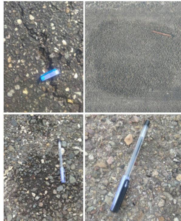
Figure 3: Some Photographs from Distress Survey at Simara Airport, clockwise from top left: 8H, 10L, 11 and 12H
